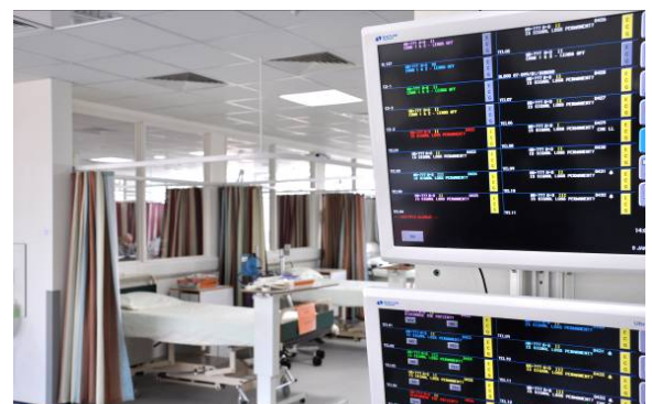
Central monitoring and ECG telemetry on all beds
